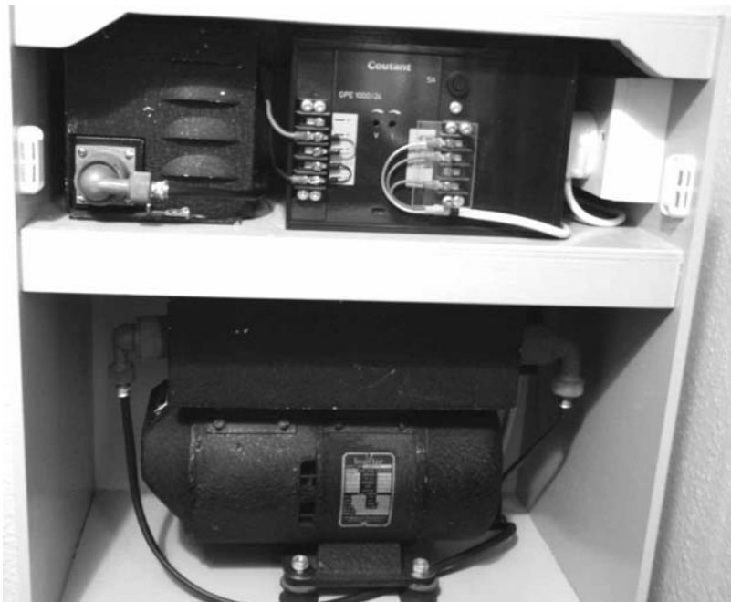
Fig 2 Main power supply consisting of an 800W rotary inverter.
